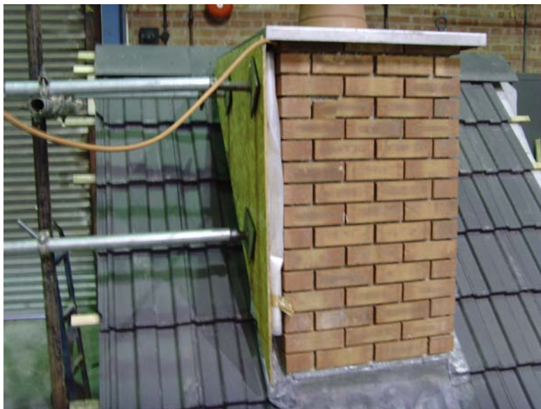
Plate 4 General View of Mono-pitch Chimney under Wind Load
